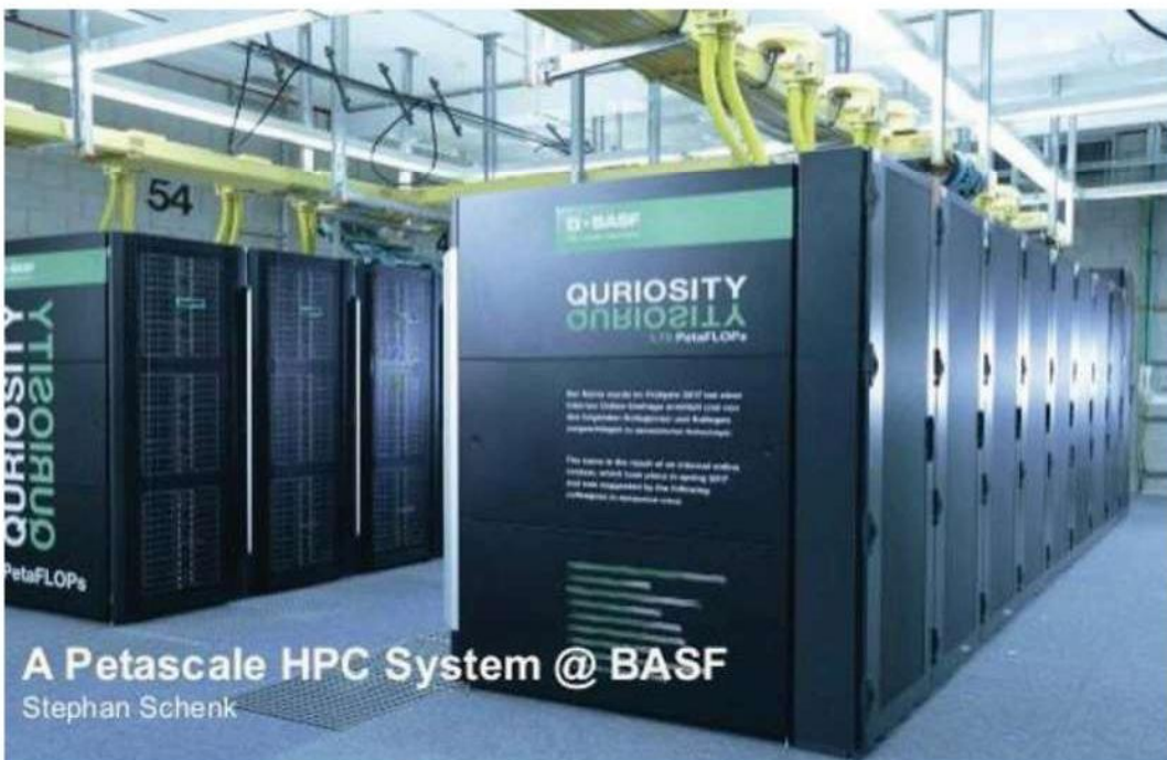
BASF High-Performance Computing Cluster
